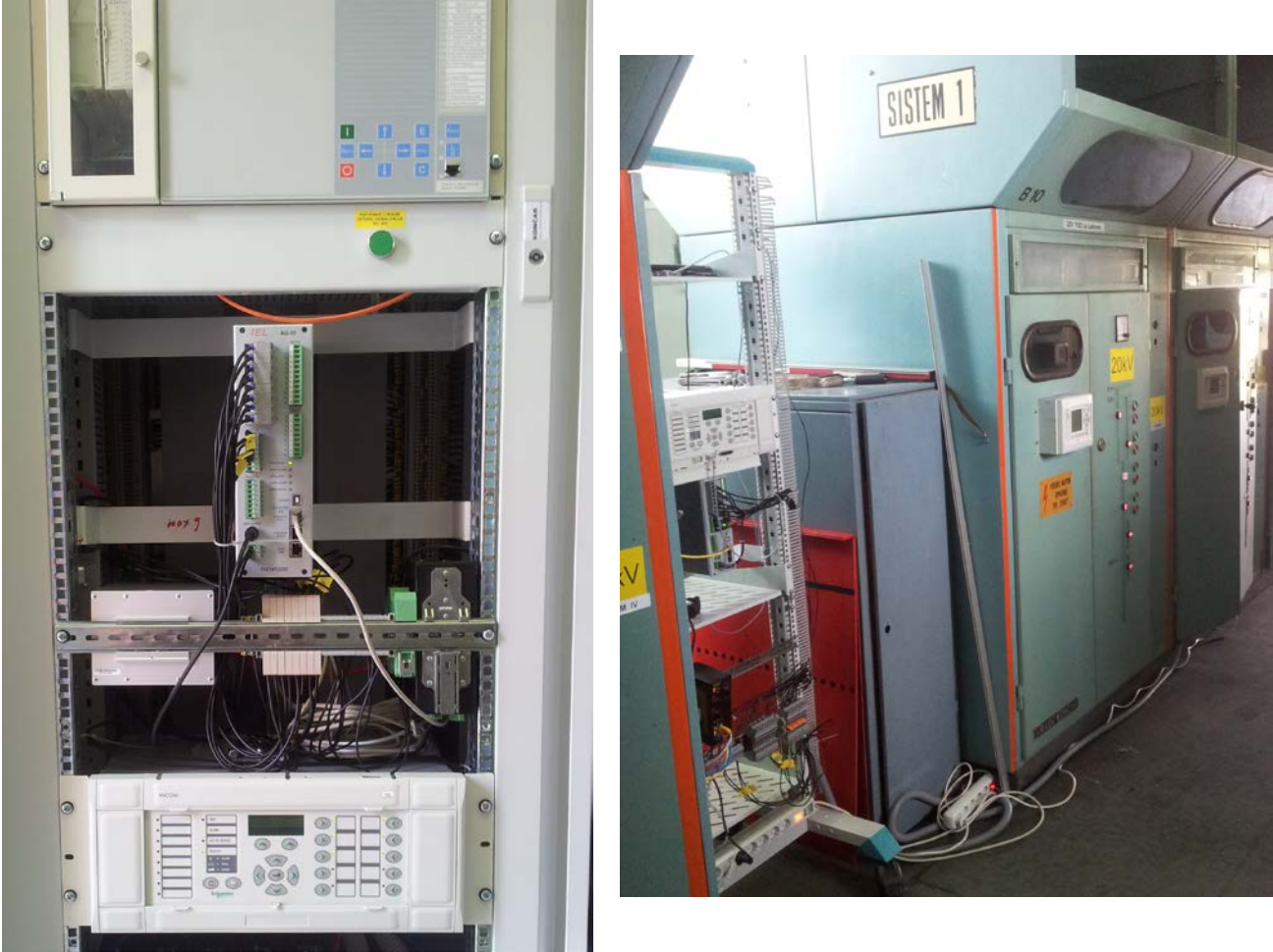
Figure 4 Installations of SAMU pilot projects on left side 110kV and or right 20kV OHL
