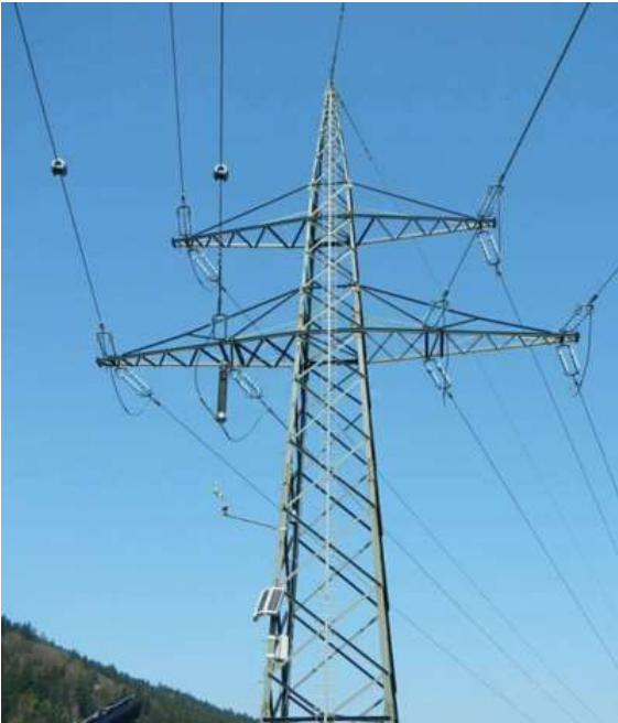
Figure 5: Standard configuration of the OTLM system – weather station and 2 x OTLM
