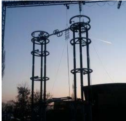
Fig. 3 Knee type disconnecter 1000-1200kV project – Outdoor dielectric test set-up
