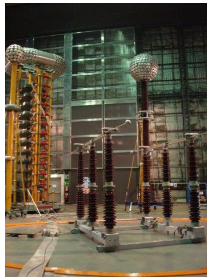
Fig. 2 Two pole disconnectors with double open gap - set up for dielectric test
