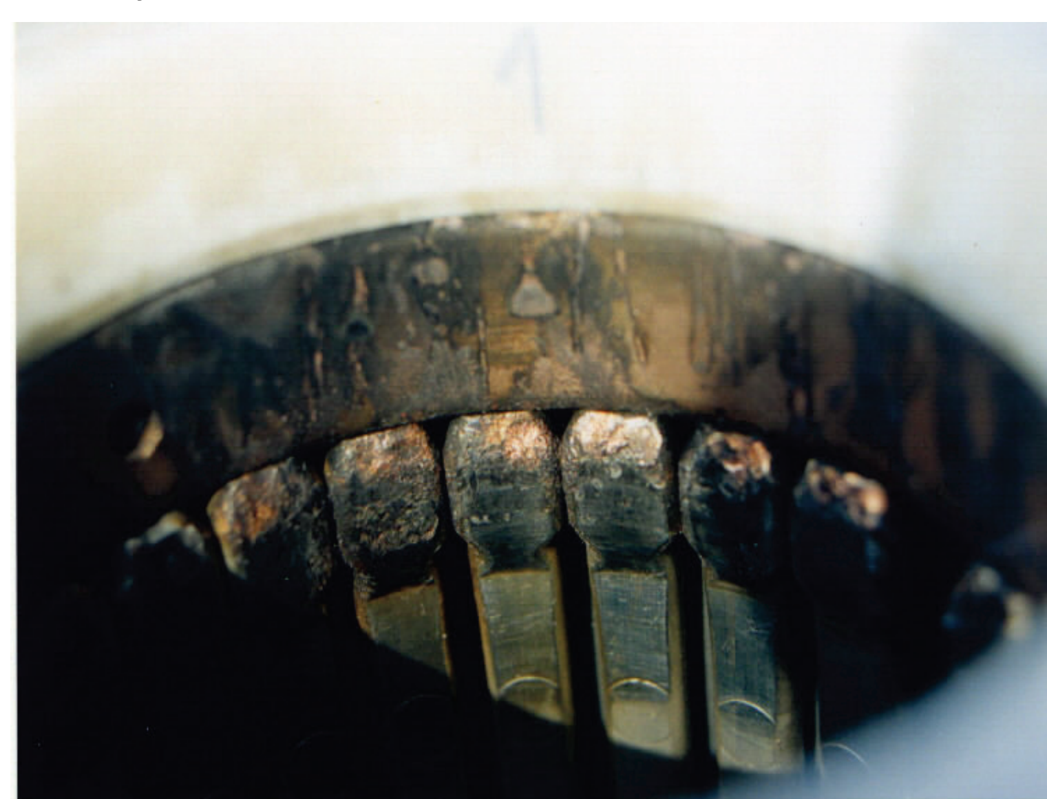
Figure 2: Damaged contact system.
