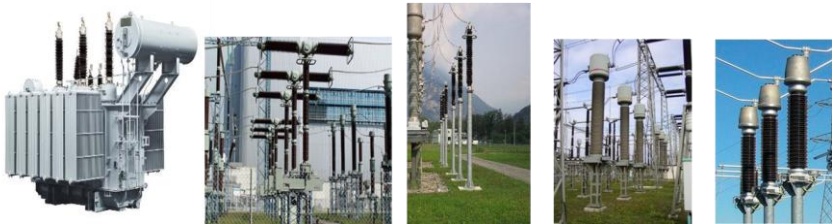
Figure 3: High voltage substation equipment
