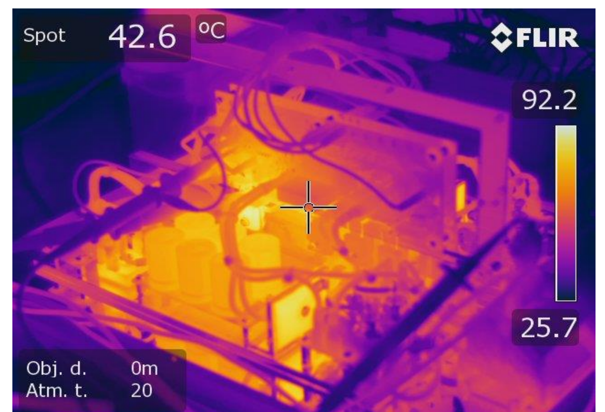
Circuit thermal testing
