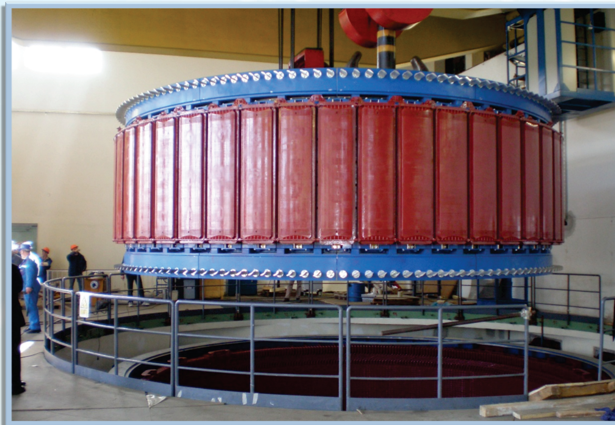
HPP Zlatoličje upgrade from 74 MVA to 85 MVA
