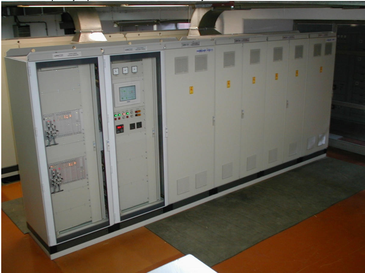
Figure 5 New Končar excitation system of the synchronous generator at Varaždin HPP, Croatia
